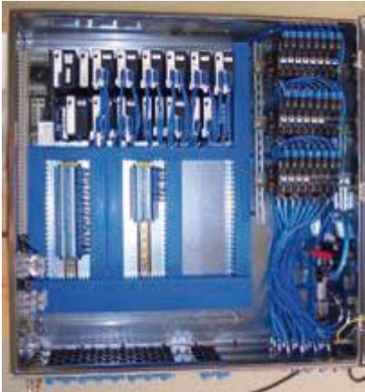
Fig. 3: Remote I/O Zone 1 field cabinet solution
