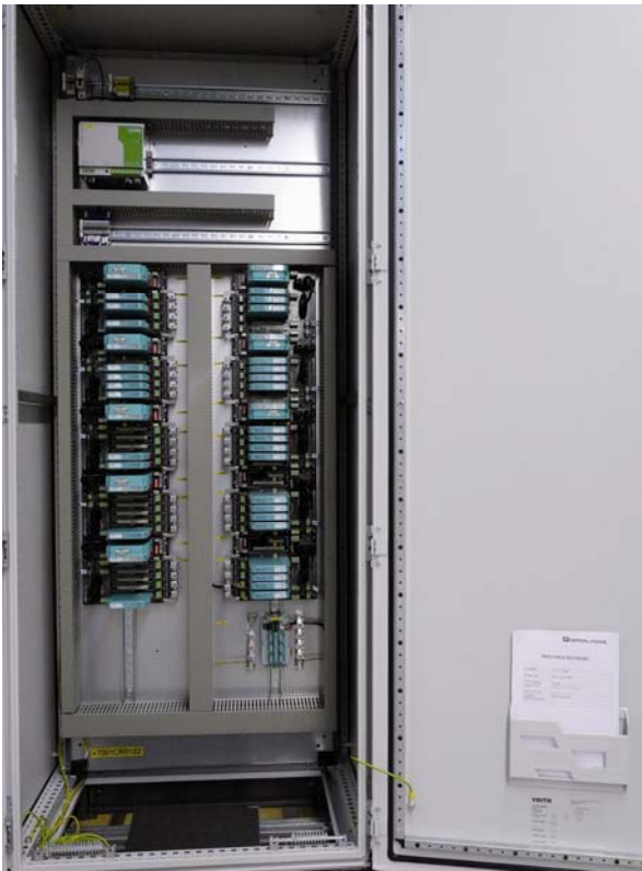
Fig. 1: Fieldbus Power Hub Cabinet
