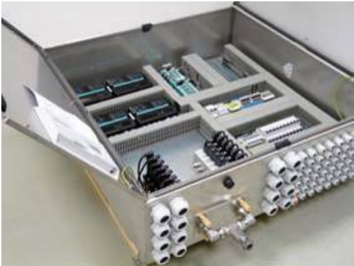
Fig. 2: Field Distribution station with Segment Protector, valve coupler and low power valves
